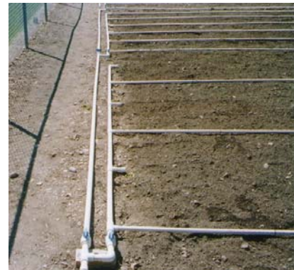
Main distribution line is glued, lateral lines are not glued
